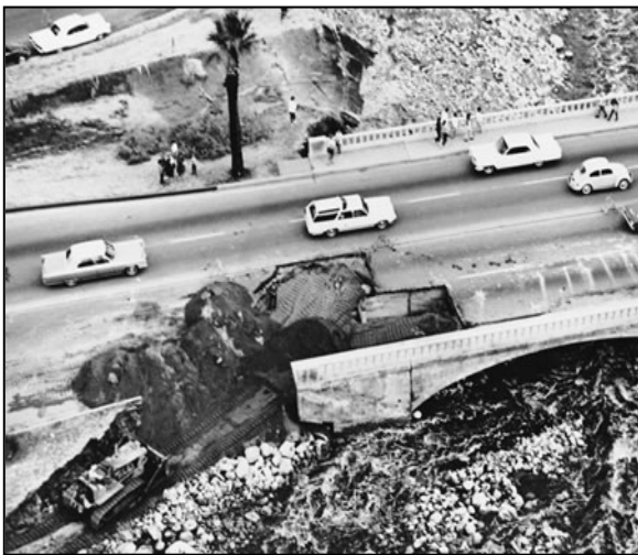
Flood damage to Highway 111 from 1965 storms.
