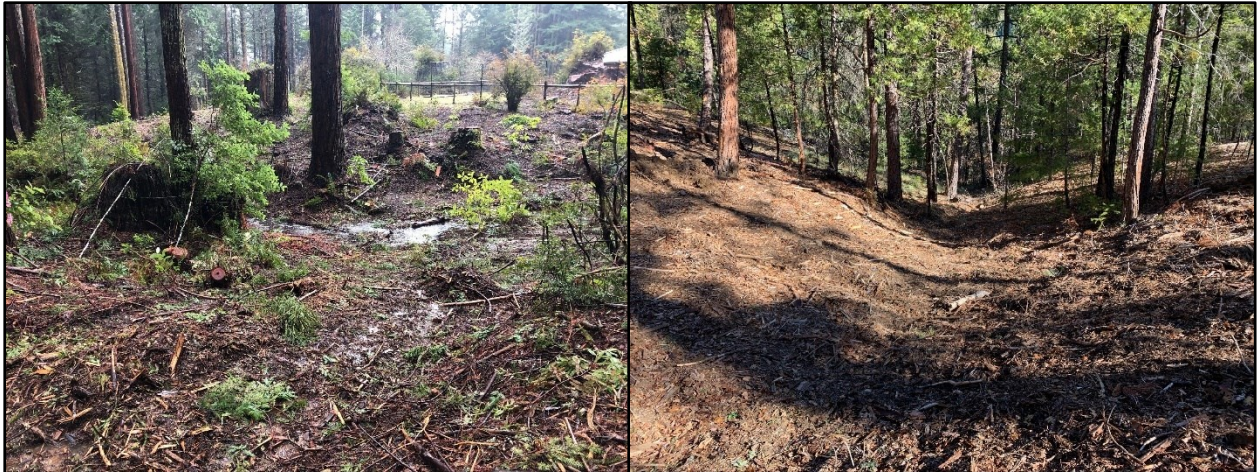
Figure 7: Skid trail crossings of Class III watercourses, with “Trace” sediment discharges. The left photo shows what was an unmapped Class III that was flowing during a rainfall event, while the right photo shows a Class III that had a temporary crossing, with waterbarred and slash packed skid trail approaches (not shown).
