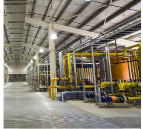
Yucaipa Valley Regional Water Filtration Facility treats 10 million gallons a day.
