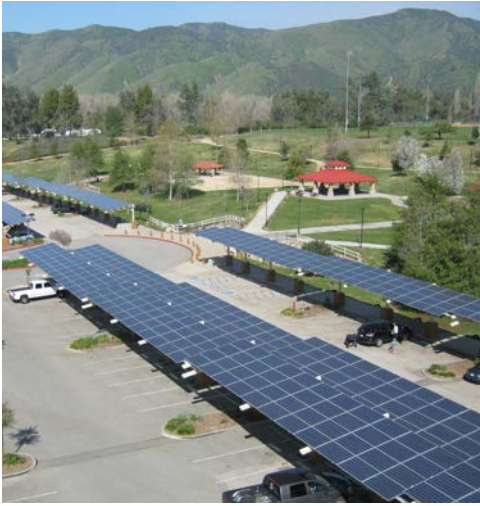
Solar panels at Yucaipa Community Park are part of the City's efforts to conserve and produce clean energy.
