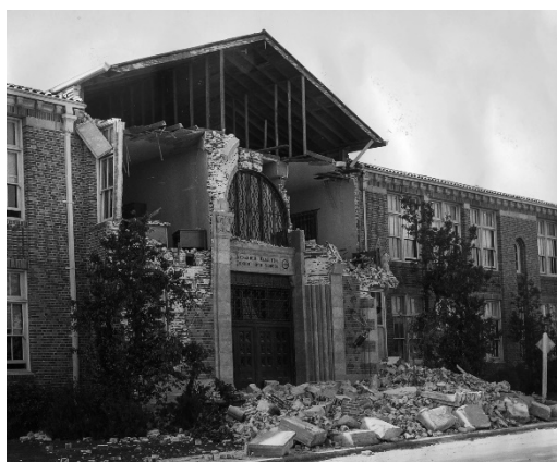
Seismic shaking primarily affects unreinforced masonry buildings, as seen here with this Long Beach middle school damaged by the 1933 Long Beach earthquake. Image from Los Angeles Times.
