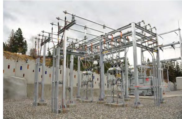
Electrical substations are vital facilities to ensure that electrical service is safe and reliable. Image from Paul Chernikhowsky.
